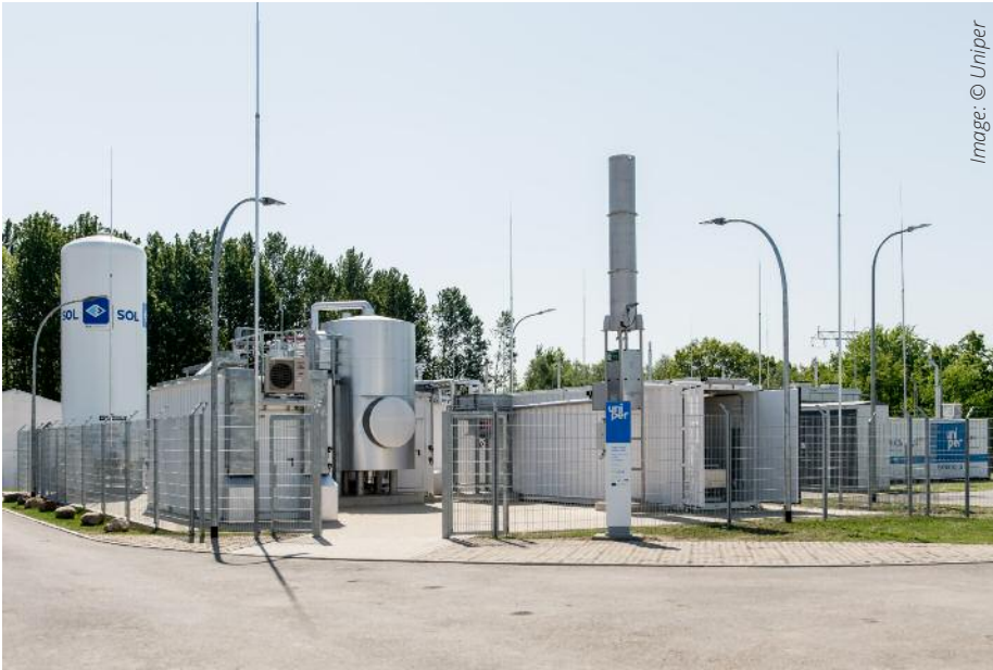
One of STORE&GO's three demo sites: Methanation demo plant in Falkenhagen, Germany, with the rounded methanation reactor at the centre (© Uniper)
